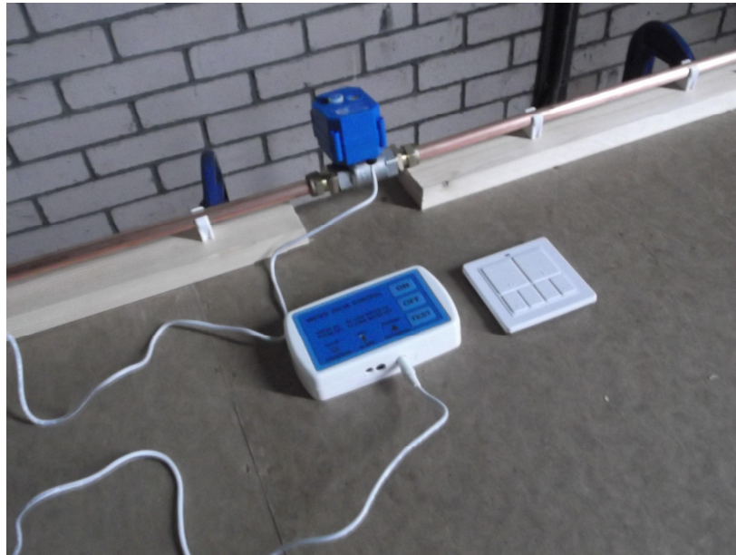
Photograph 6: LeakSafe set up for manual remote switching on and off the water supply (water stop valve connected to valve control unit)
