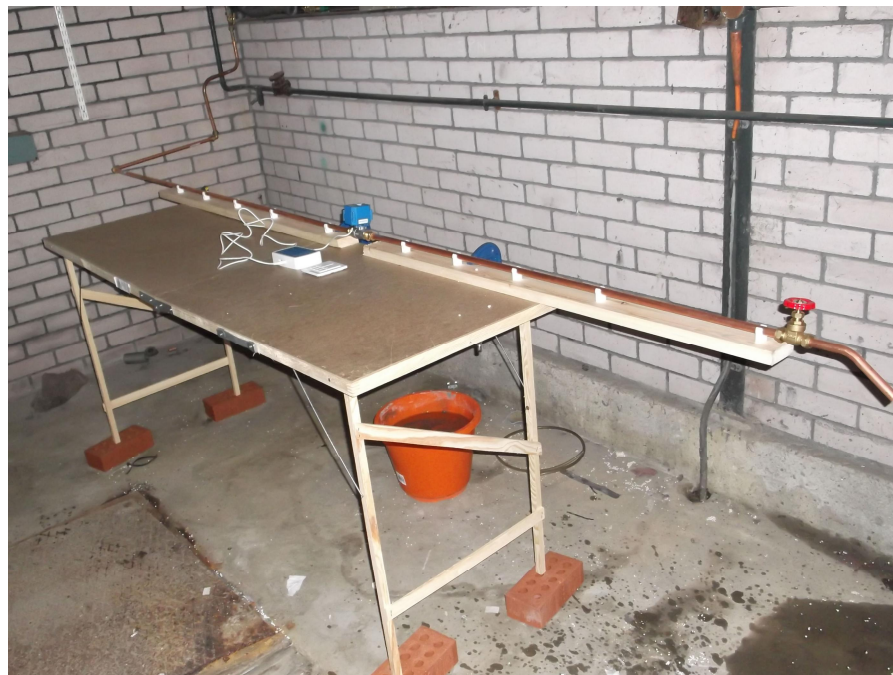
Photograph 5: LeakSafe water stop valve fitted to 15 mm water supply pipe
